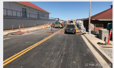
Crews installing and compacting road base material, laying asphalt and striping pavement
